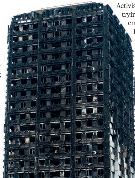
● Grenfell Tower in the aftermath of the fire
